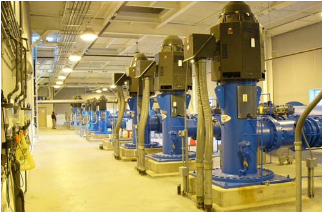
Cooling Water Pump, 30HXB
